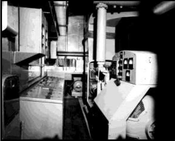
The generator room
