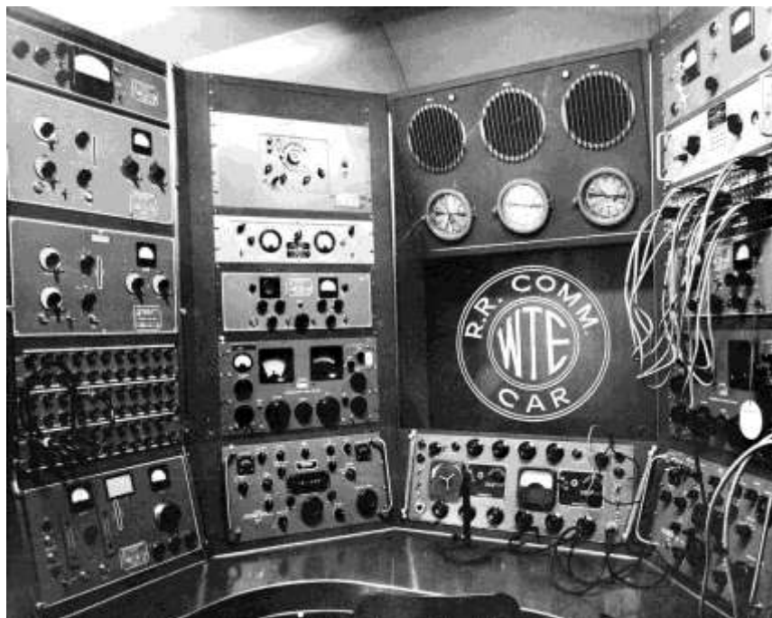
Above radio control console occupies part interior of presidential communications General Myers Car. Multiple control panels, a maze of gadgets for radio broadcasts, radio photo
